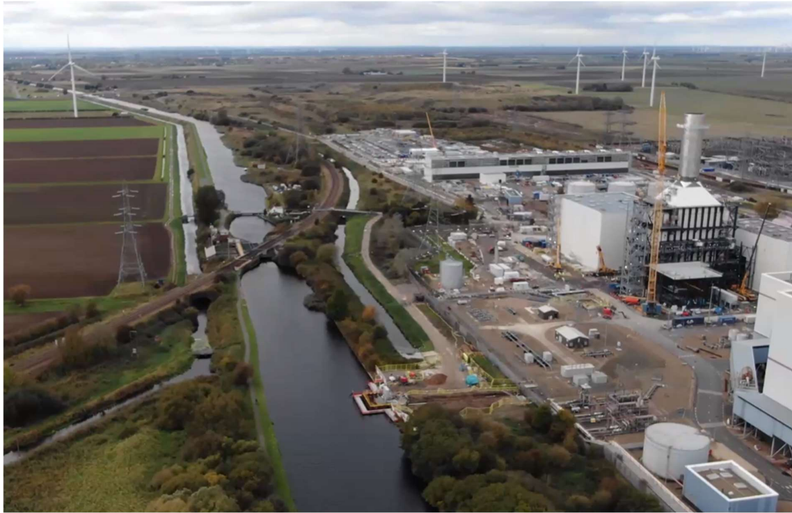
Photograph 19 – Aerial view of the construction area for the Keadby 2 Power Station water intake on the Stainforth and Keadby Canal, drone footage taken November 2020
